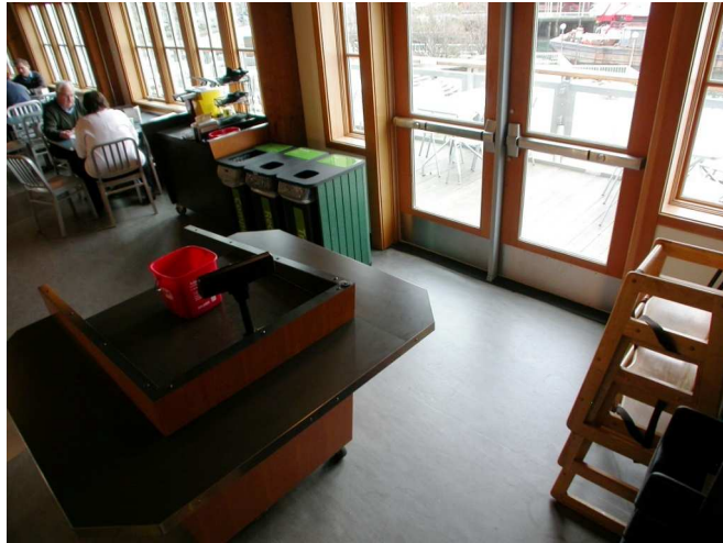
Figure 10: Accessibility Issues at Exterior Balcony Door
